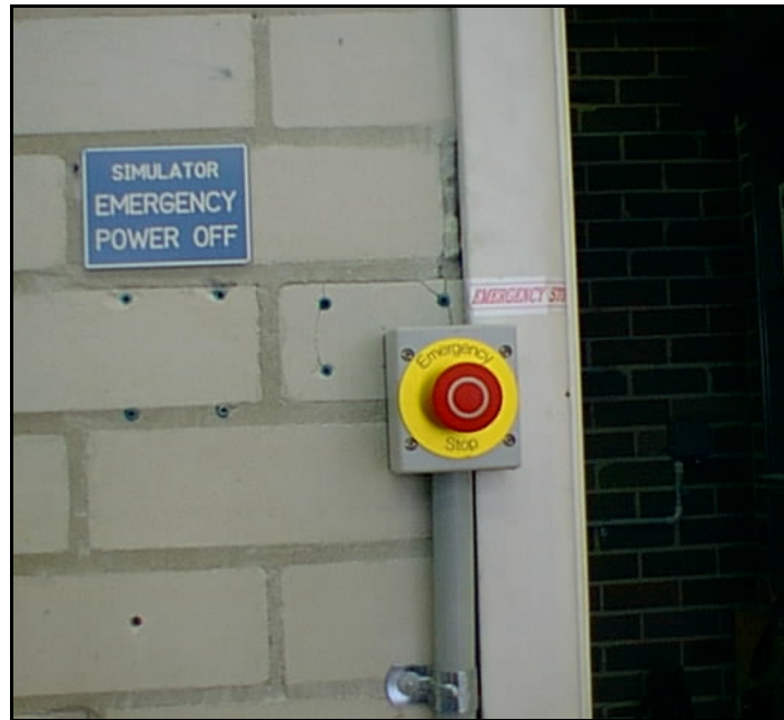
Figure 78 HPU Emergency Stop Switch
