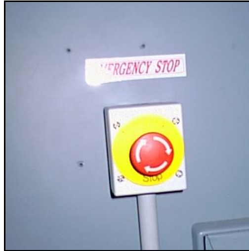
Figure 77 IOS Emergency Stop Switch
