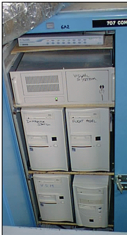
Figure 48 Main Computer Cabinet
