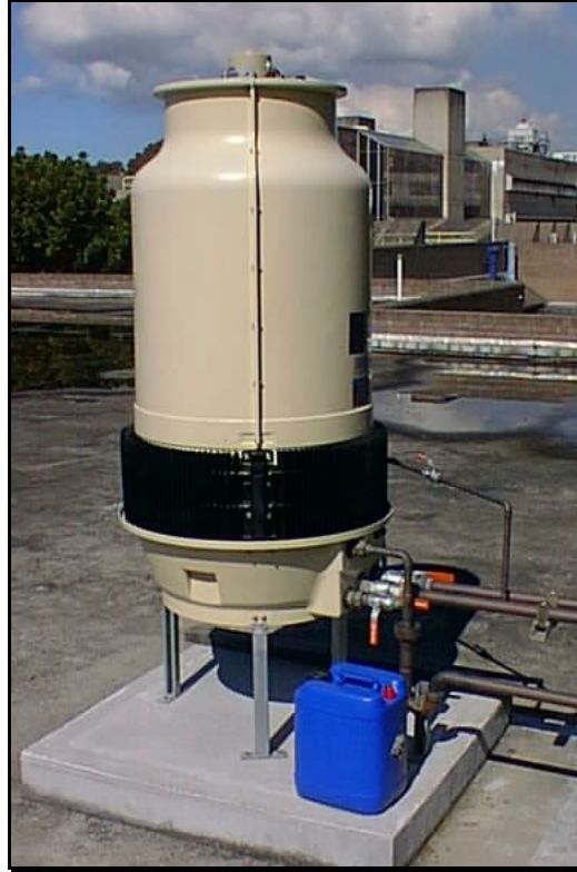
Figure 33 Shinwa SBC10 Cooling Tower
