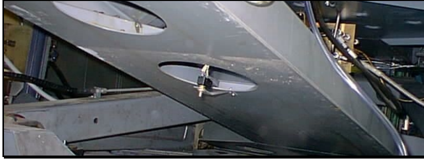
Figure 59 Safety Circuit Nose Switch
