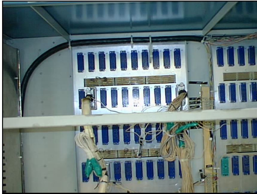
Figure 24 The Junction Box
