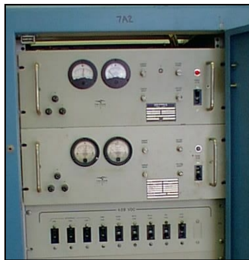
Figure 31 DC Power Supply Controls
